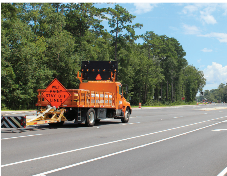
Road resurfacing and pavement evaluations are two major projects that will take priority in Bryan County in 2022.
