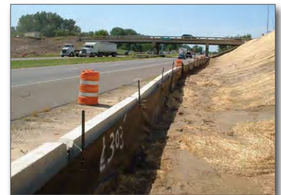
Figure 20. Silt fence protecting a highway and underground fiber optics cable
