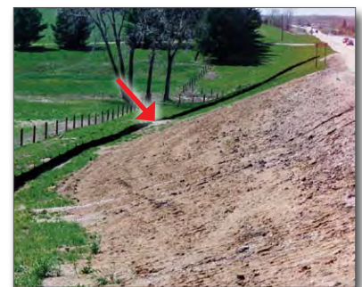
Figure 4. Avoid long runs of silt fence
