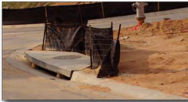
Figure 7. This silt fence doesn't work
