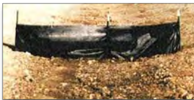
Figure 9. Poor installation, water can flow around the ends causing additional erosion
