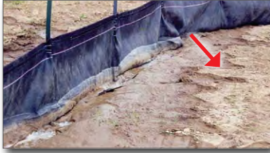
Figure 16. Poor compaction has resulted in infiltration and water flowing under this silt fence causing retained sediment washout
