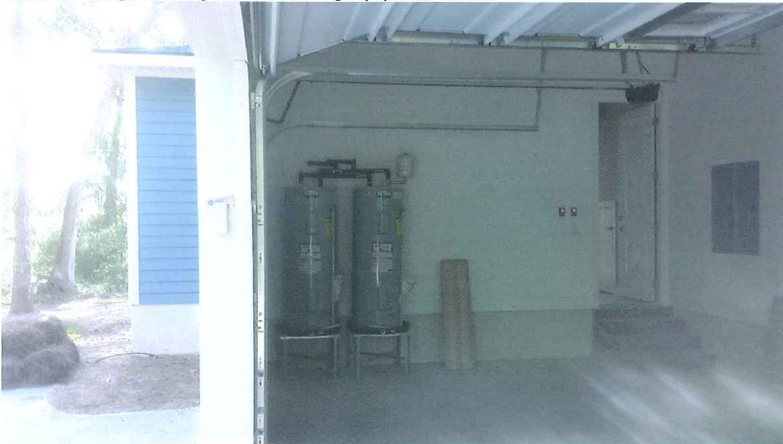
Inside of Garage showing lowest servicing equipment for C2e
