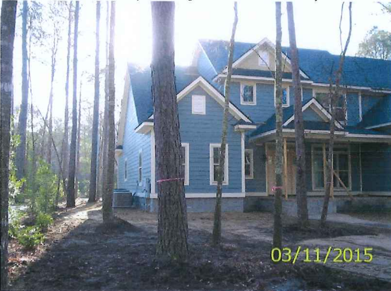
Front - Left Side View (showing A/C for section C2e)
