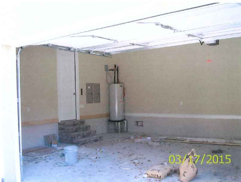
Inside garage showing showing lowest servicing equipment – C2e
