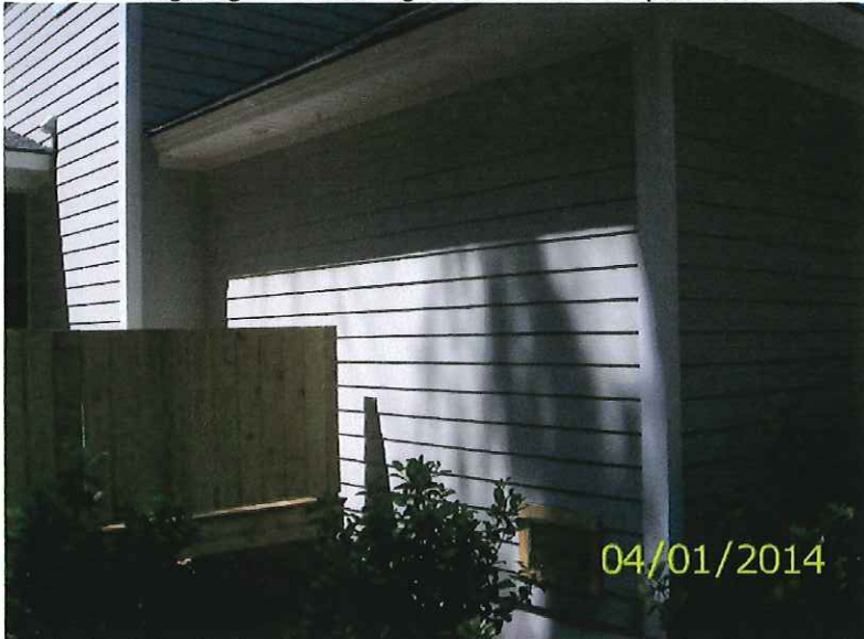
Left Rear of garage #2 showing Smart Vent. A/C platform on left
