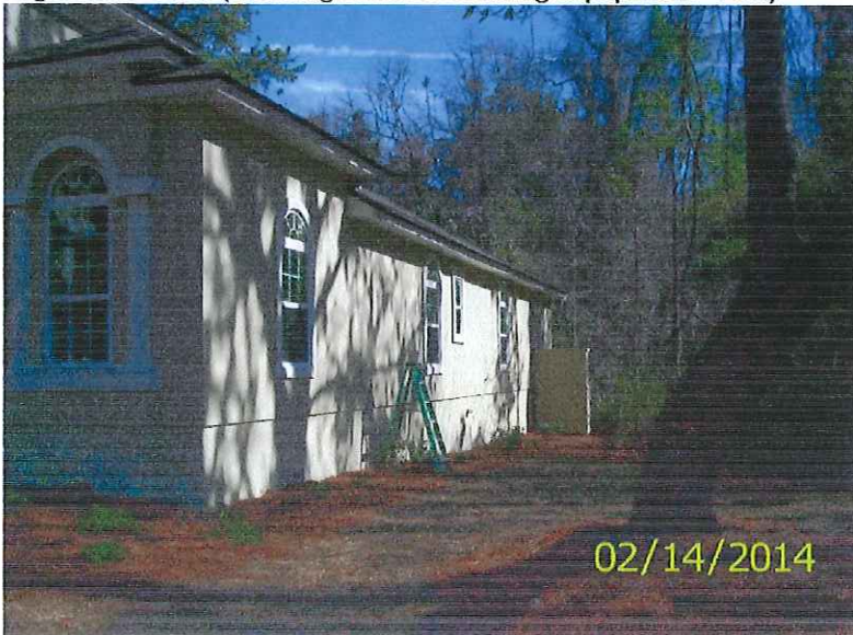
Right Side View (showing lowest servicing equipment - A/C)
