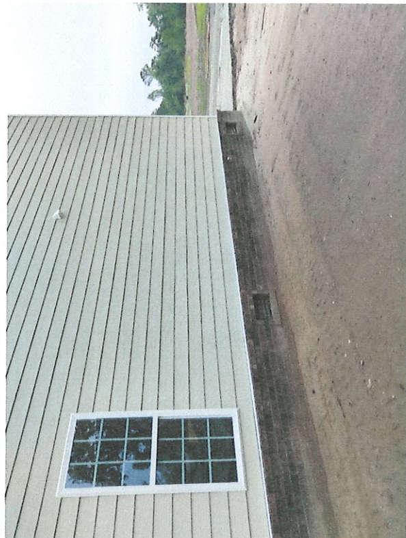
Rear View taken 4/23/2018 showing the lowest servicing equipment for C2e
