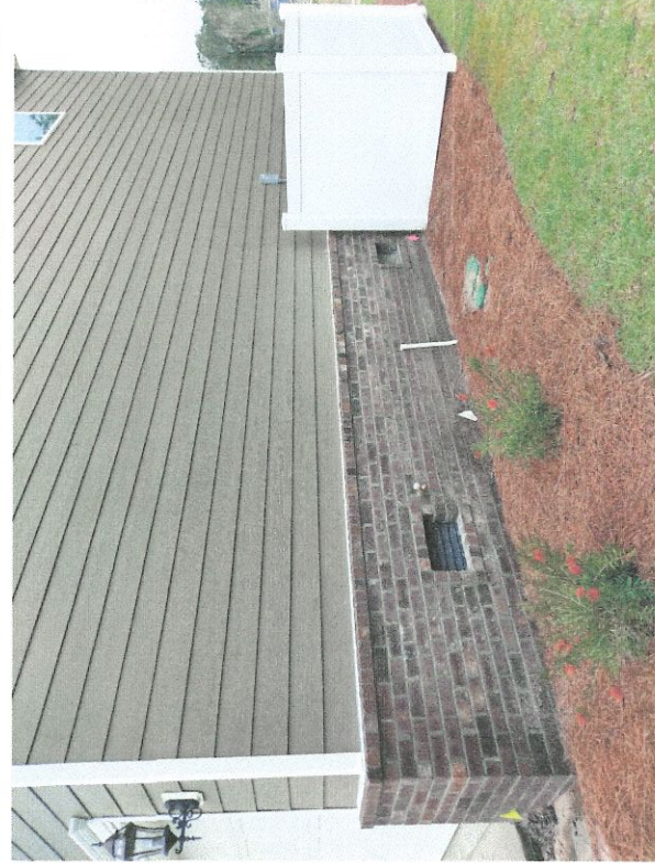
Rear View taken 4/23/2018 showing lowest servicing equipment for C2e
