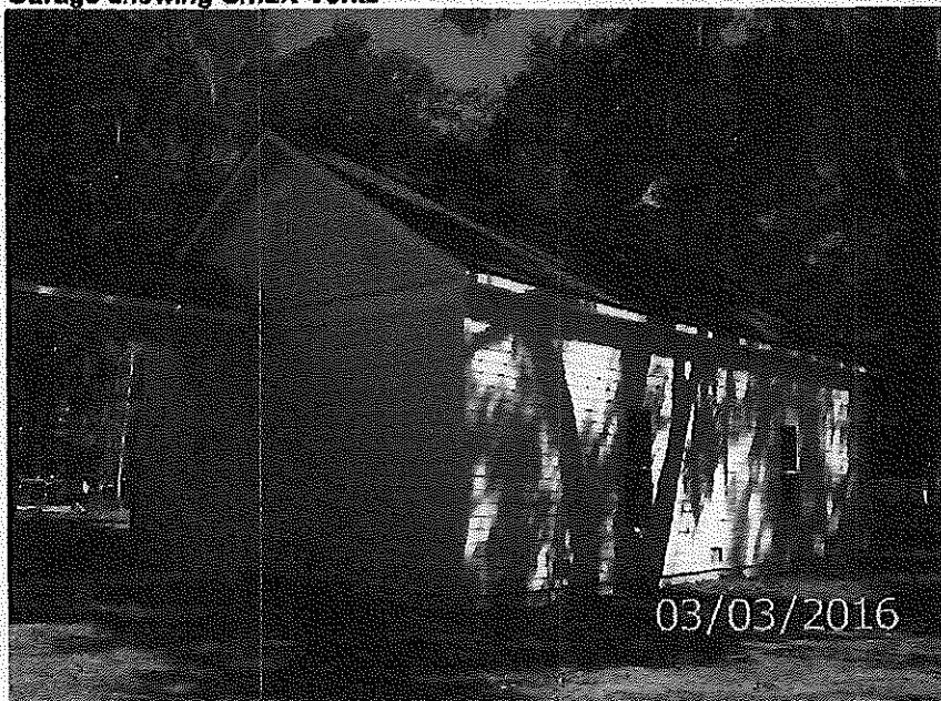
Garage showing Smart Vents
