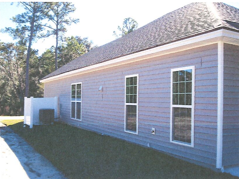
Right Side View taken 1/8/2020 showing lowest servicing equipment for C2e
