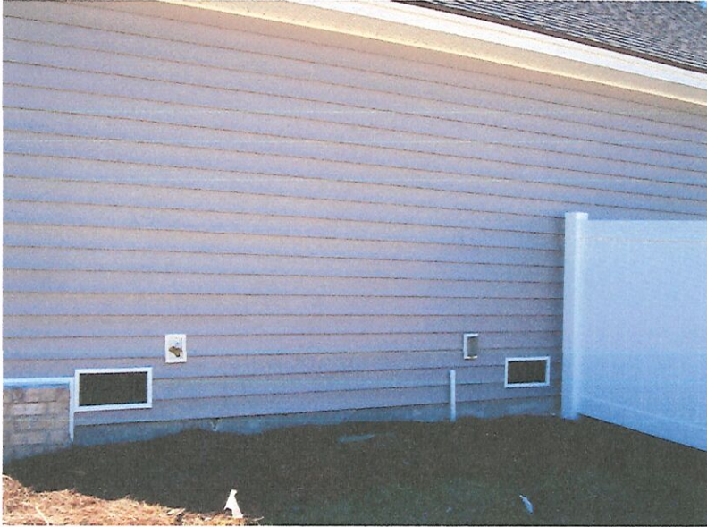
Right Side View taken 1/8/2020 showing engineered flood vents
